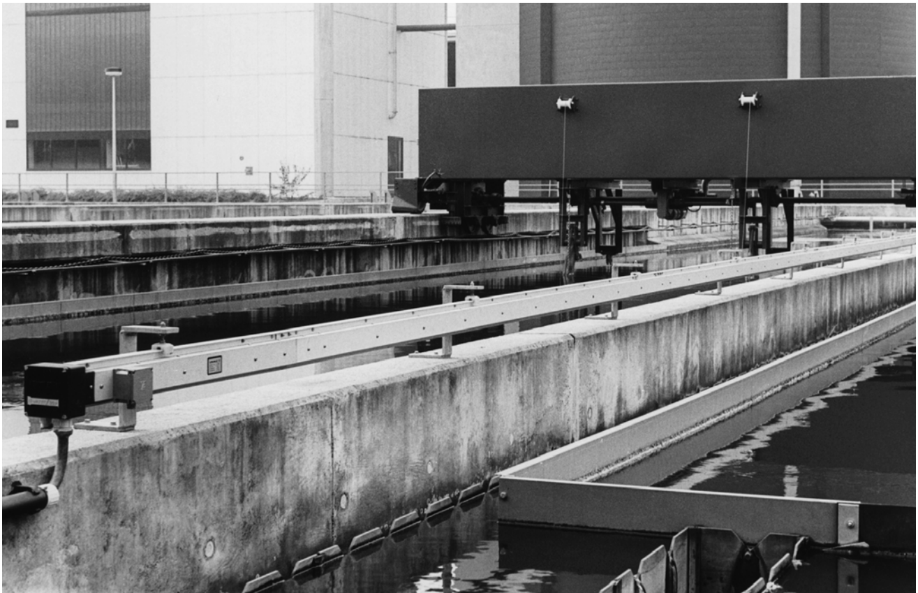
LSV Powerail feeding sewage treatment system
