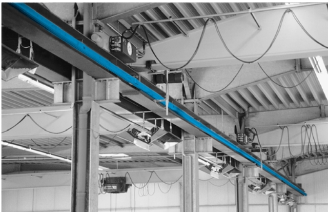
LSV serves for OHT crane electrification
