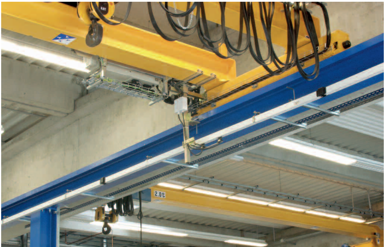
Crane installations at company Rheinmetall Landsysteme (Kiel)
